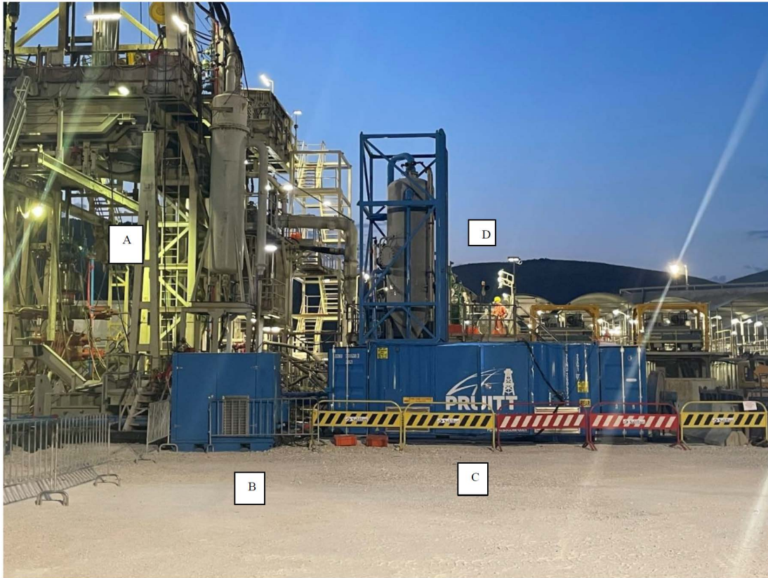
Figure 2—MPD System Rig up with A- RCD Bowl, RCD Bearing, HCR Valves and pipework, B- MPD Transformer skid, C- MPD Choke Container, D- ASME VIII U Stamped Mud Gas Separator (MGS) (16 ft liquid leg, 30 psi MAWP) with real-time level monitoring and alarms
