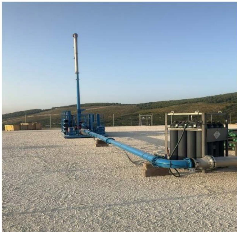
Figure 3—Pruitt Flare Stack (30 ft) with Flame Arrestor and Real time Gas Flow Meter
