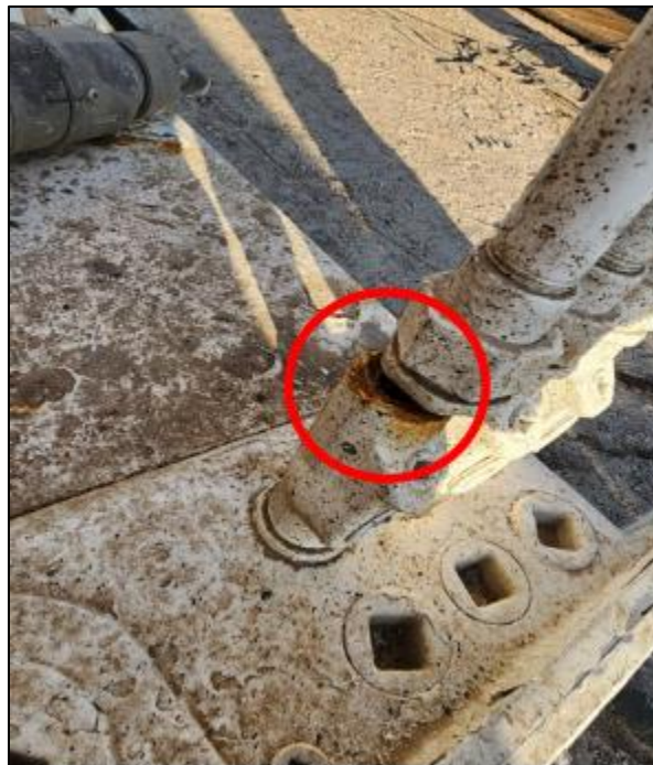
Area of damage to the unit allowing moisture inside once the silicone was removed from this area.
