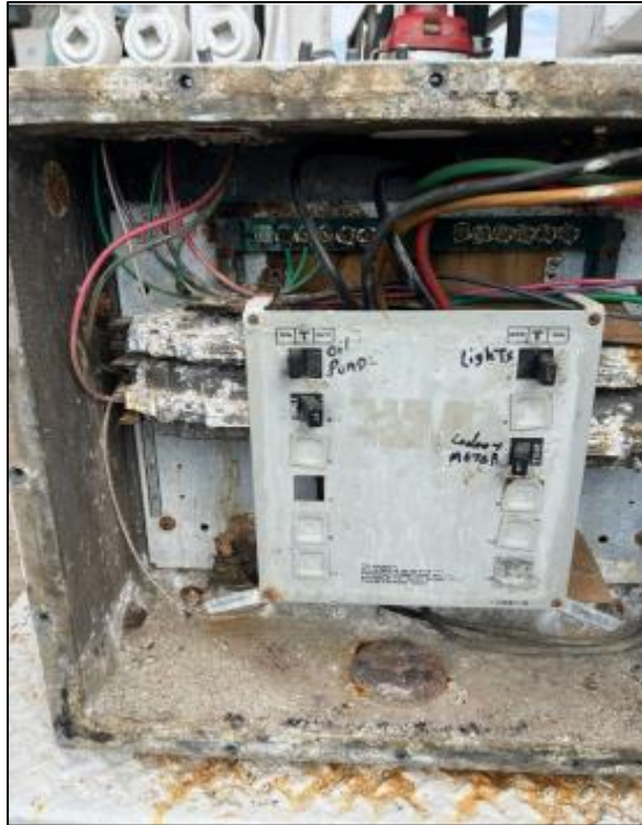
Showing breaker panels inside unit.
