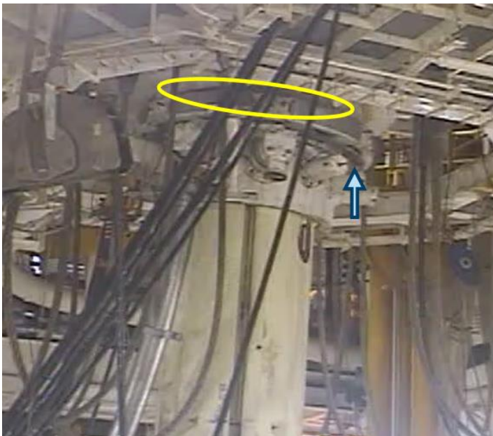
Fig-2: Screenshot from CCTV. During pulling of the BOP through the splash zone a gap between tension and gooseneck ring emerged, as indicated by yellow circle
