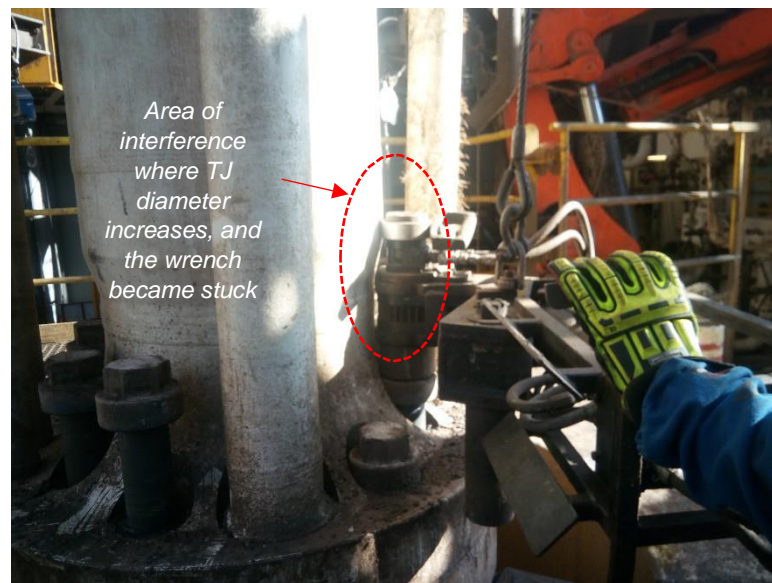
Reenactment of the position of the Riser Torque Wrench on the Telescopic Joint (TJ)
