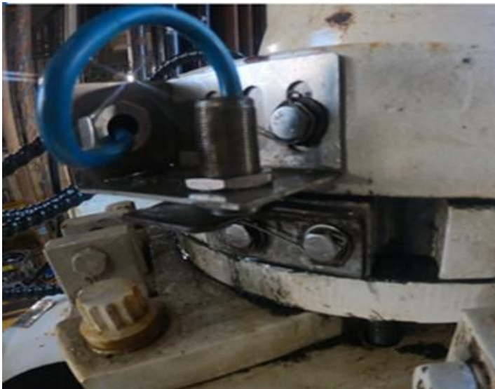
Figure 2 Proxy Switch giving signal to driller when the RRT is locked
