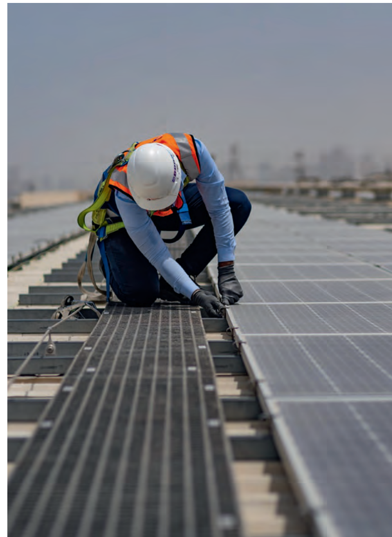
Maintenance of solar panels on the rooftop of Emirates Glass in Dubai.
