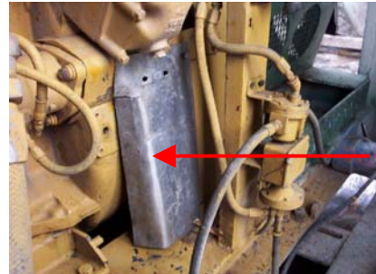
Fabricated guard to eliminate access to exposed Fly wheel and clutch.
