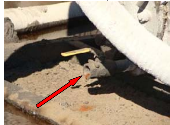
Figure 5 After fleet wide distribution of the initial issuance of this safety alert, the pump was corrected by removing the bull plug and adding a new ball valve lever.
