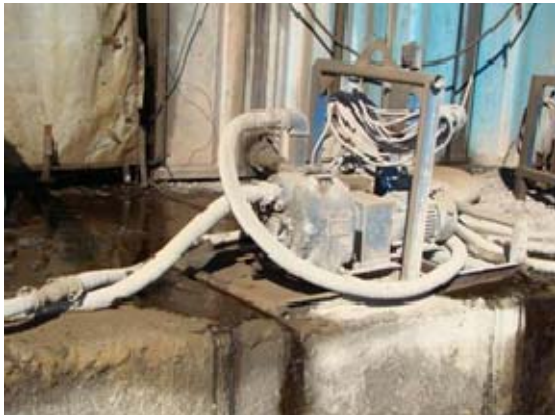
Figure 4 Follow Up Inspection 2 months later on same transfer pump from which the safety alert was initiated (see next picture).
