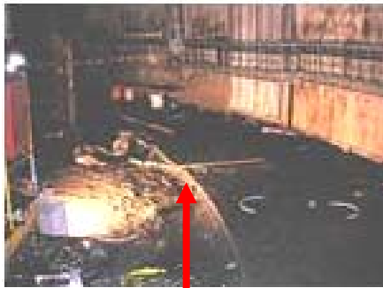
A board covering the manhole. The incident area in similar lighting conditions
