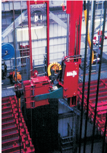
Maritime Hydraulics' Configurable Automatic Drilling System (CADS) will be installed on BP's Valhall platform in the North Sea. The bridge crane and fingerboard are pictured above.
