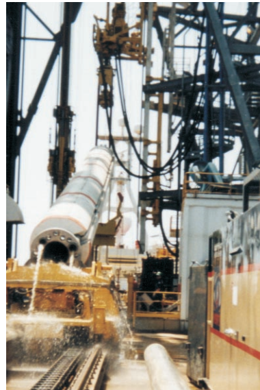
The riser was being run from the C.R. Luigs in early May in 6,700 ft of water.
