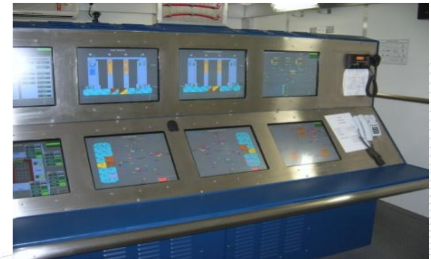
MPMS CONTROL ROOM – SEMI-SUBMERSIBLE UNIT
